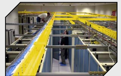
M2M data center hosts the application and data, and around-the-clock monitoring from a network operations center ensures maximum availability, backup, and automatic recovery – providing the basis for guaranteed service.
