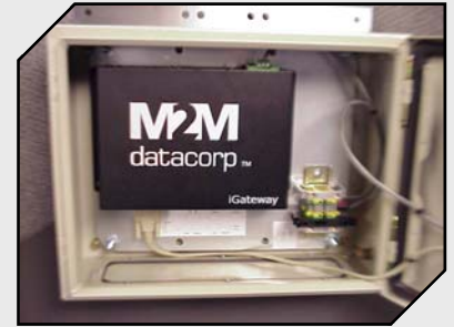
M2M iGateway’s link compressor control panels into an IP satellite network. NEMA-4 enclosures endure extreme exposure to the elements.
